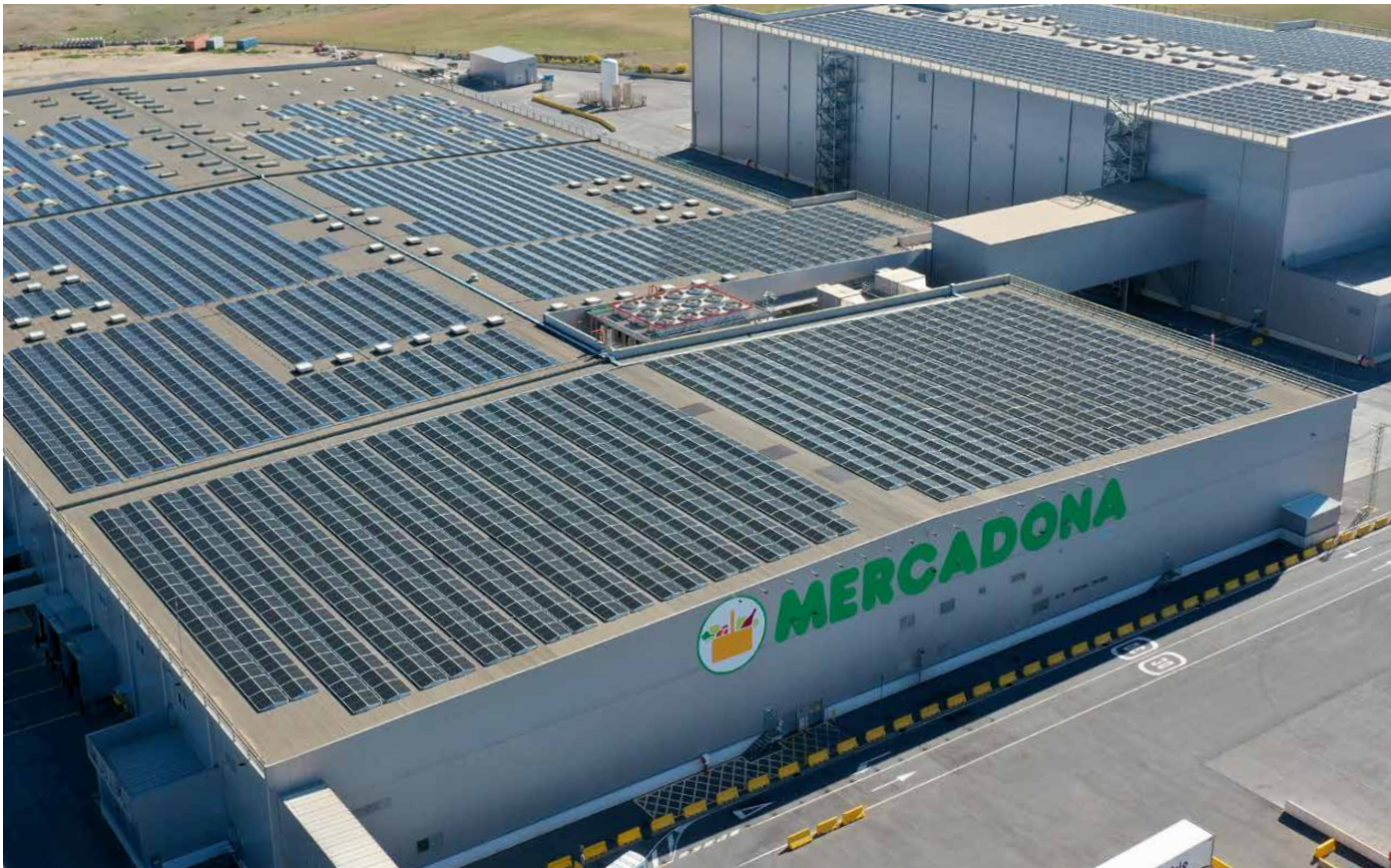
Solar panels installed at the logistics centre in Guadix, Granada.
